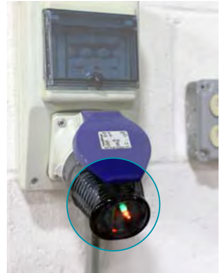
GREEN & RED LAMPS LIGHT One phase is missing
