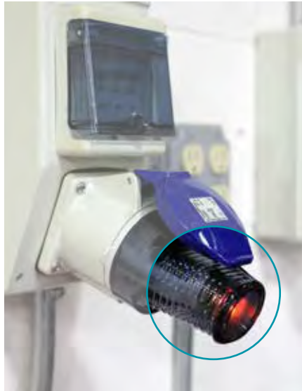
RED LAMP LIGHTS Phase sequence is wrong
